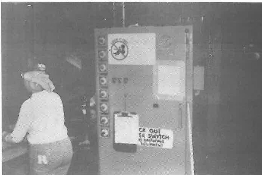
Figure 3. Sign warns workers and repairment to lock-out equipment before performing maintenance or repairs.
