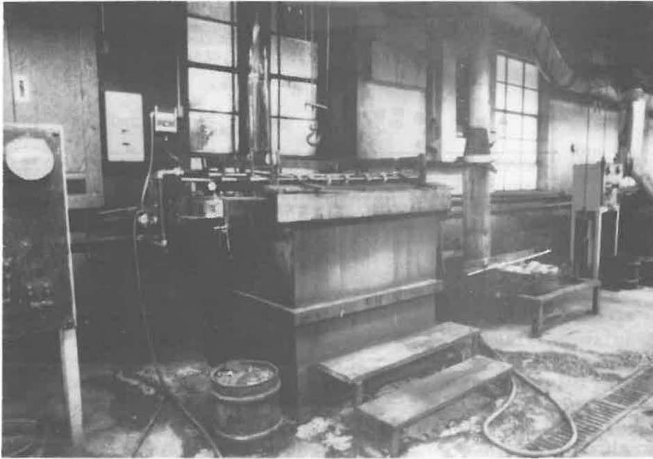
Figure 6-5. Tank - three-sided ventilation.
