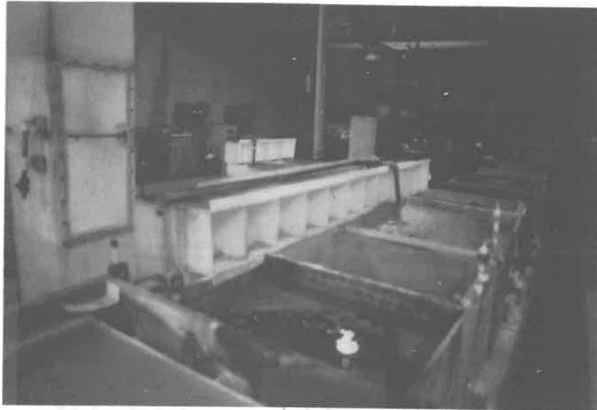
Figure 6-25. Acid cleaning line and exhaust hood.
