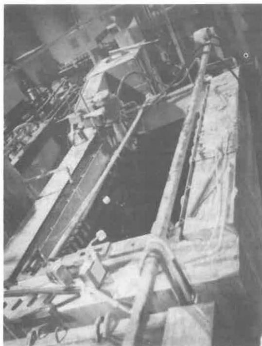
Figure 6-22. Cadmium plating tank - ventilated.
